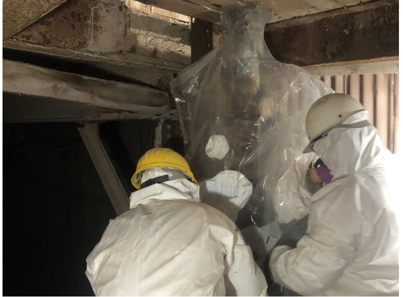
Asbestos removal: "Glove bags" rap around a historic pipe to seal in asbestos while workers put their hands inside the built-in gloves to remove fibers safely.
