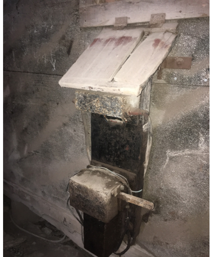
Signal switch by the Lander's office of the shafthouse
